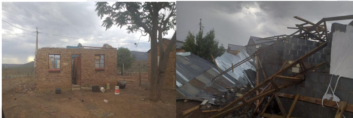
Image 1: Structural damage from the microburst (Source: Garth Sampson)
