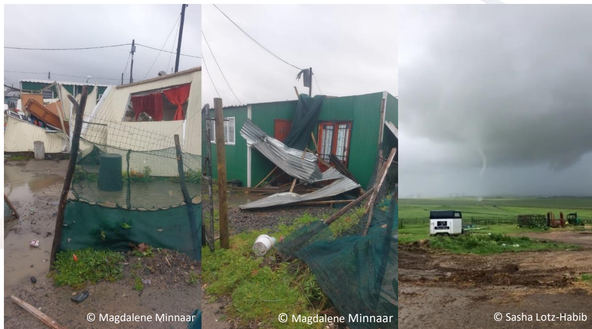
Figure 1: The damage (left and centre) due to the EF-1 landspout (right) that hit Cape Farms on Friday morning, 25 August 2023.
