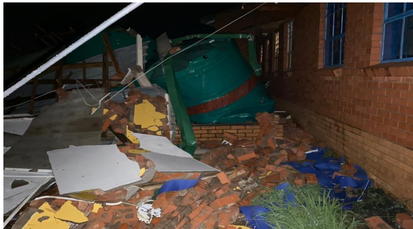
Figure 5: Collapse of a well-built wall
