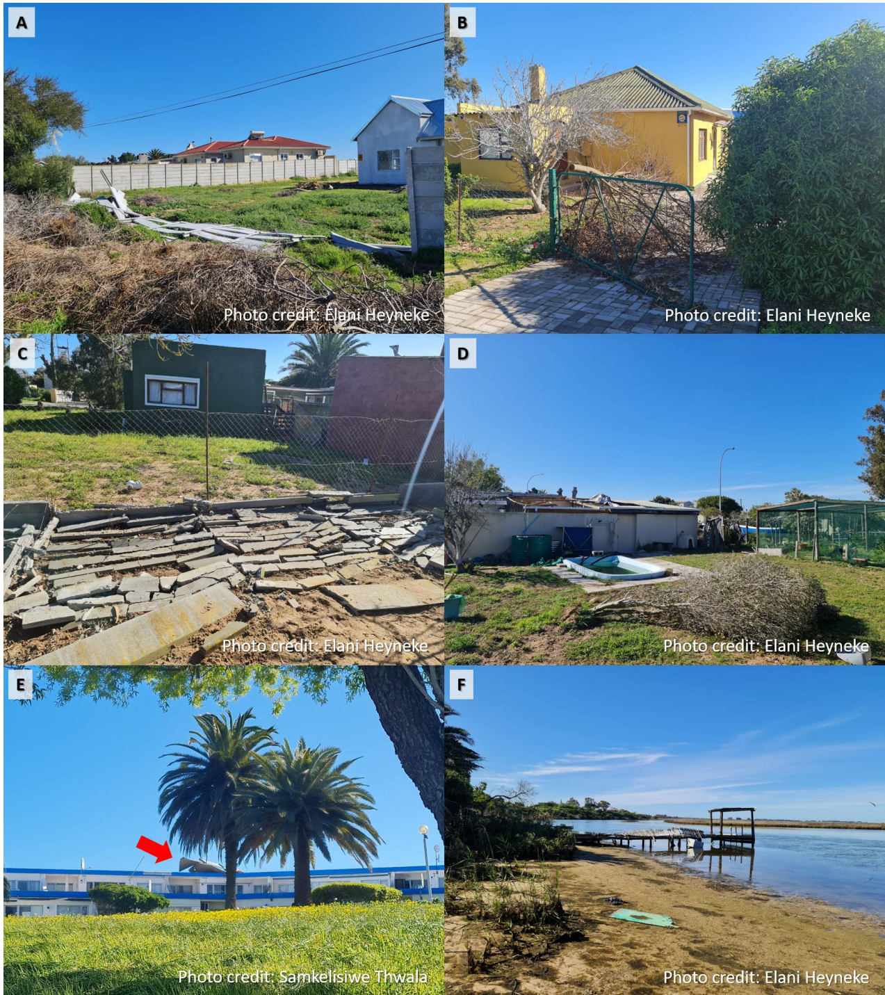
Figure 3: The damage and evidence of the track of the waterspout - the locations of A to F.
