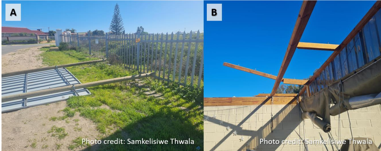
Figure 4: A) Traffic sign blown over by the force of the waterspout; B) Roof damage after the roof sheeting was taken by the waterspout.
